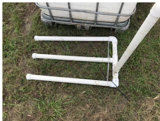
Photo 2 – Air spreader pipes
